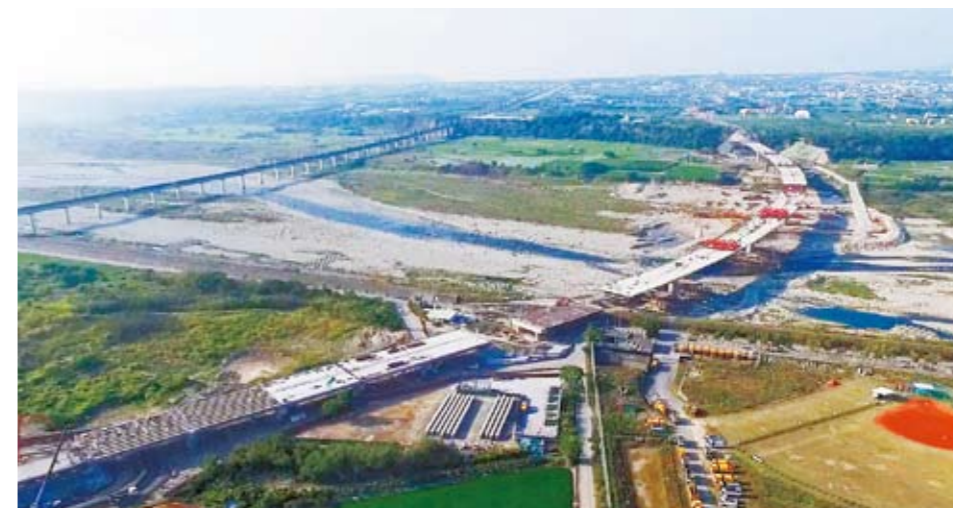
Taichung City Government strictly controlled the progress and quality of each construction at the Flora Expo. The picture shows the southbound connection highway project across the west bank of Dajia River, Yamay from the interchange system of National Highway No. 4 Shengang.
